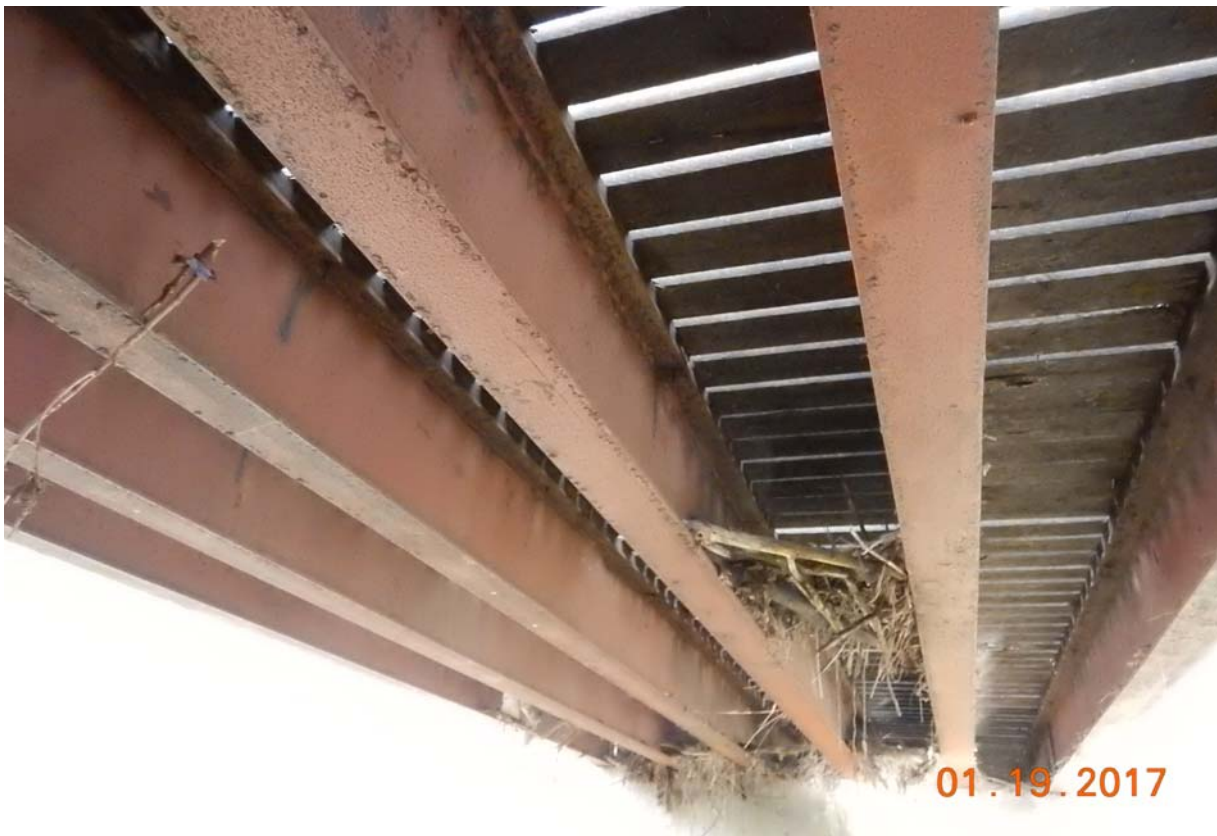
View of the underside of the east span. Note the debris lodged between the beams.
