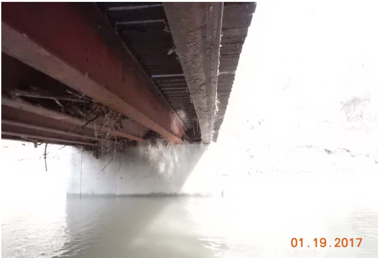
View sighting along the upstream exterior beam of the east span. Note when sighting along the beam the beam appears to be wavy.
