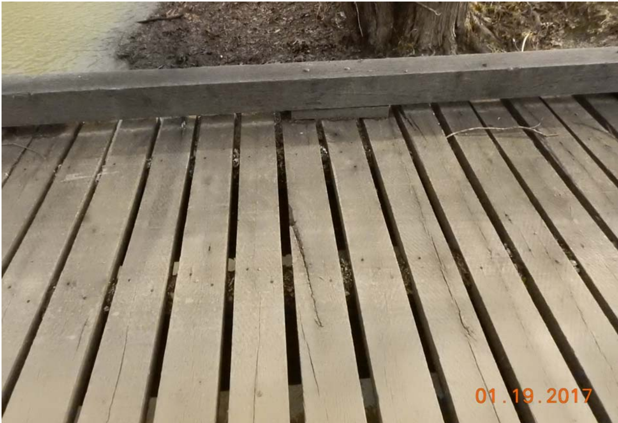
View of an area of minor splitting near the east end along the upstream wheel path.
