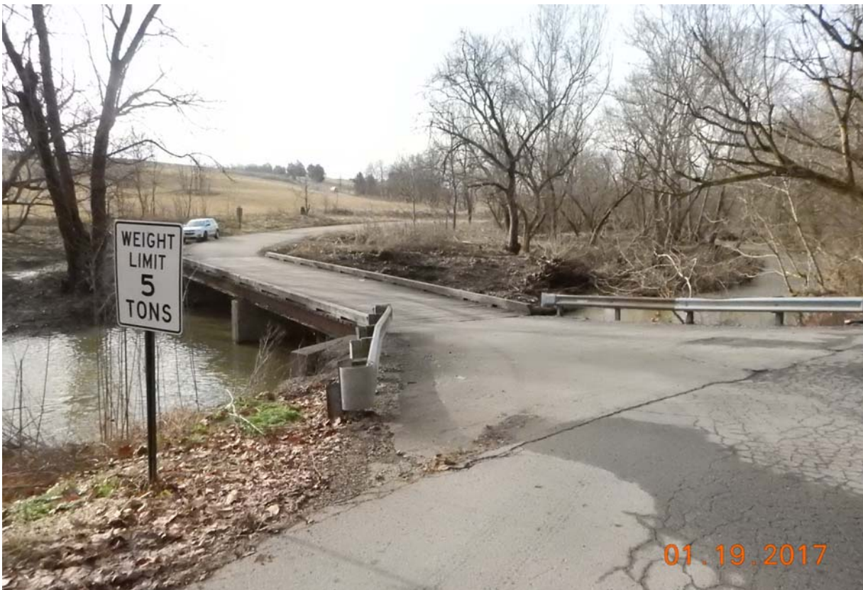
View of bridge from the west approach. Note the 5 ton posting sign is in place.
