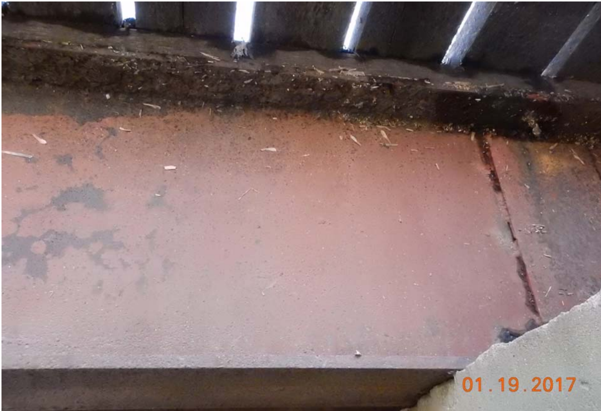
View of areas of minor pitting along the top flange of the downstream exterior beam at the east abutment.
