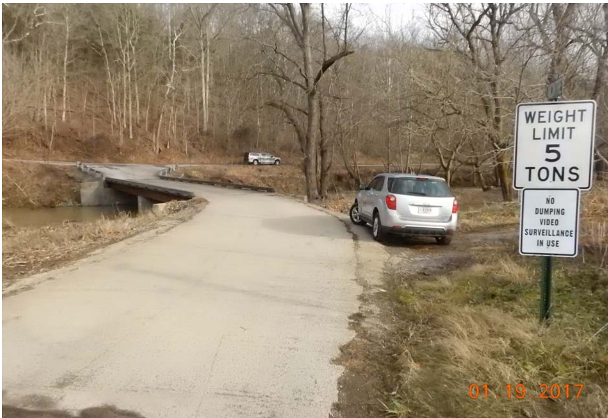
View of bridge from the east approach. Note the 5 ton posting sign is in place.
