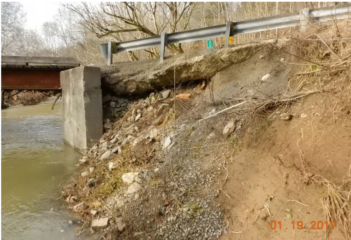
View of embankment erosion along the upstream embankment of the west abutment.
